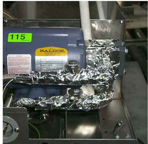
Heater strip installed [115V PF50 (Return/Suction)].
