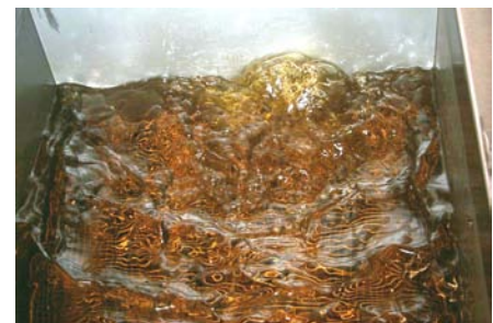
Air bubbles from the Oil Return Line
