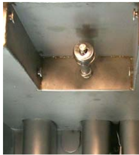
Upper float switch.
