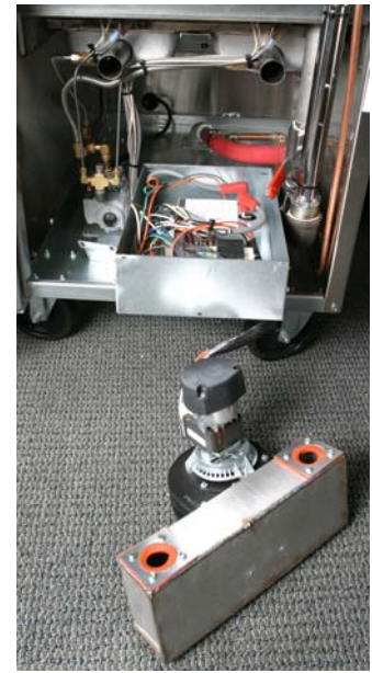
Blower and plenum removed
