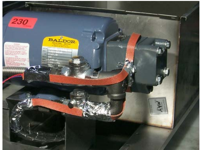
Heater strip routing on flexlines and pump [230V PF50 (Return/Suction)].
