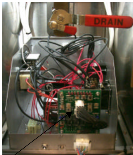
Fig: 10-7 The interface board is in the contactor box in the sub fryer.
