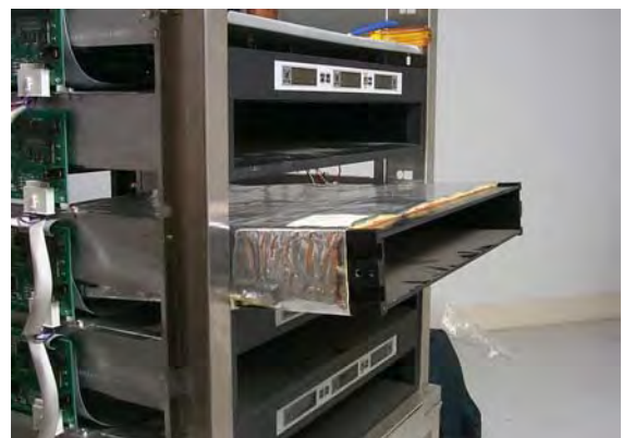
Fig. 17. Slide malfunctioning slot from cabinet.
