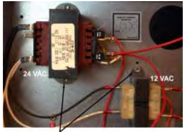
Screws securing transformers
