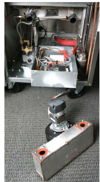
Blower and plenum removed
