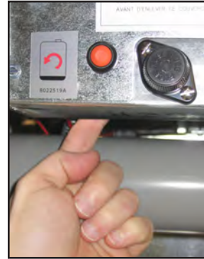
Resetting the power on an electric LOV.
