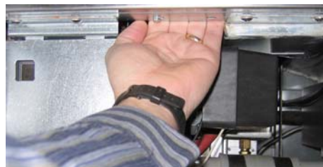
Figure 8 Resetting control power on an gas.
